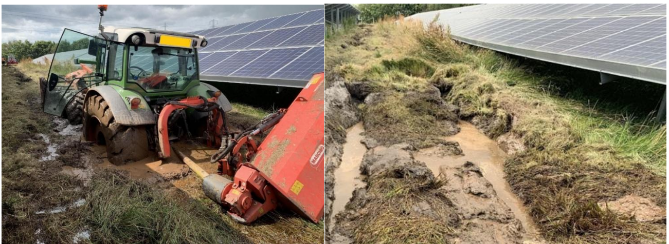
Use of Machinery in Inappropriate Conditions on silty clay based soils
